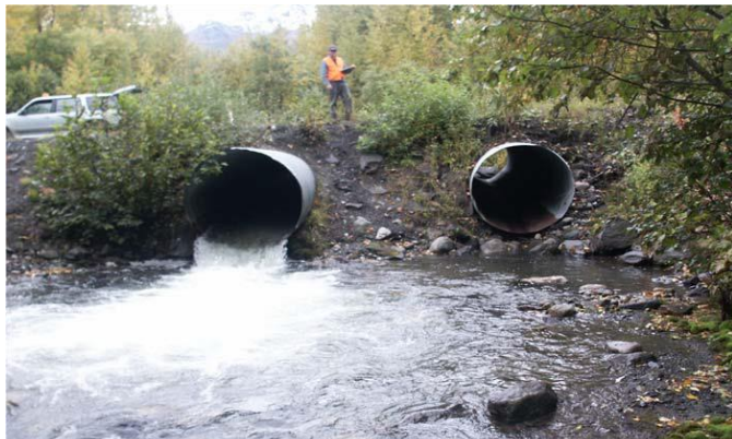
Undersized and perched culverts
