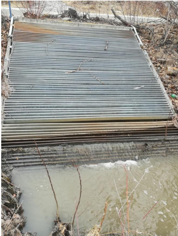
Polluted stormwater runoff being discharged directly to Lake Lucille in Wasilla.
