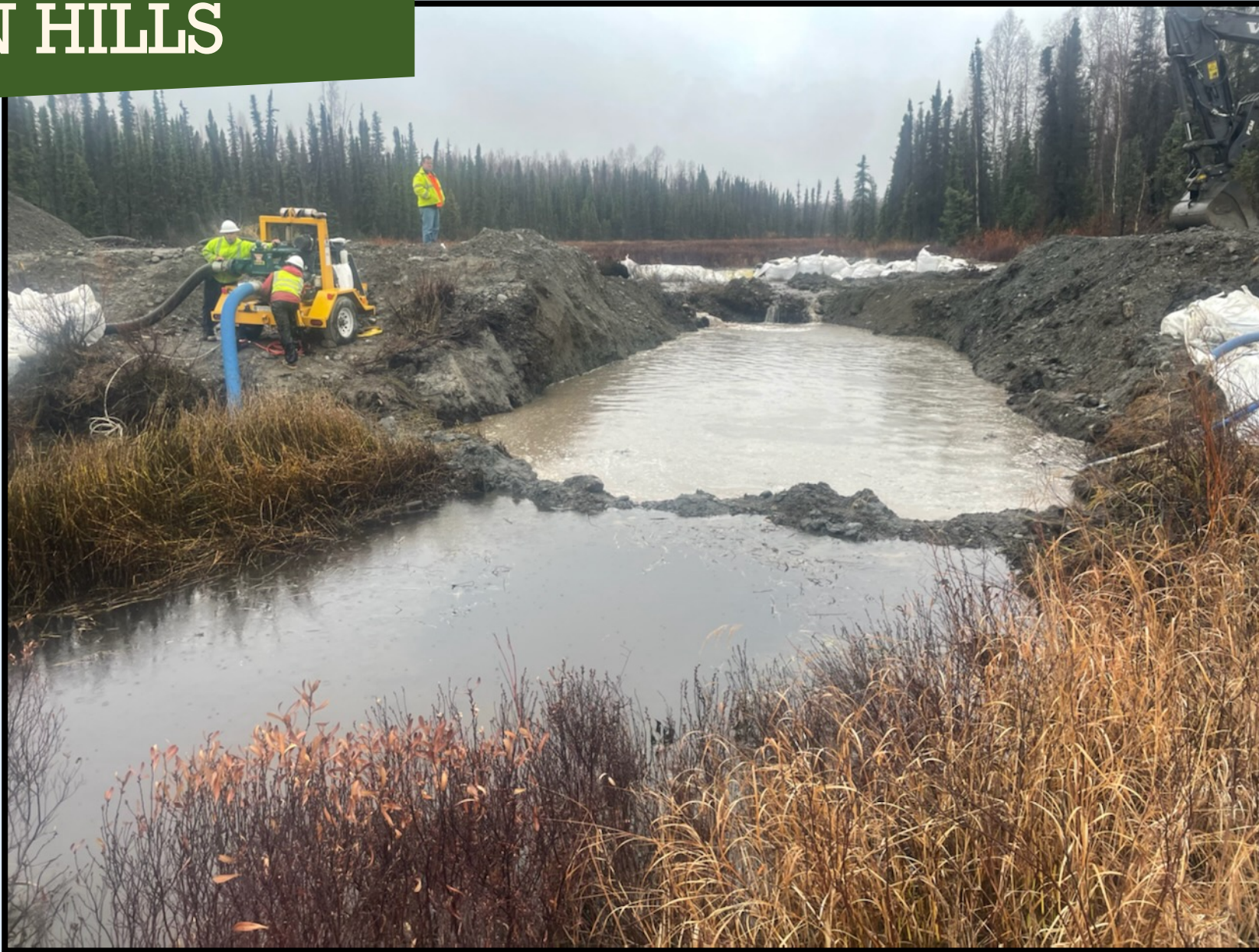
Photo: Broken cofferdam and flooded work zone.
